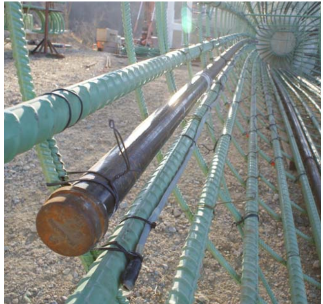
Embedded Thermal wire attached to rebar cage (shown adjacent to CSL access tubes.)
